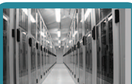
Data Center Solutions
